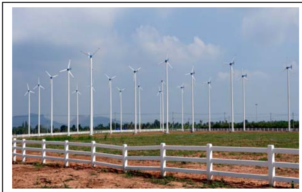
Fig. 4 100 kW mini-wind farm for grid connect
